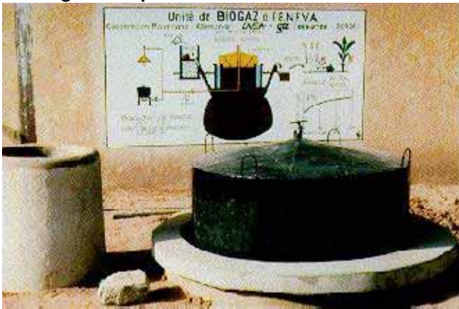
Figure 7: Floating-drum plant in Mauretania
