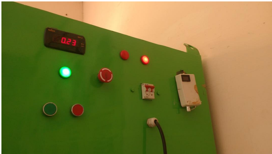
Figure:3 Control Panel
